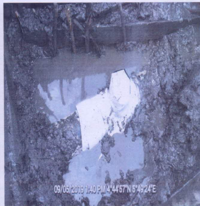
Fig D: Incident Facility shortly after repairs
